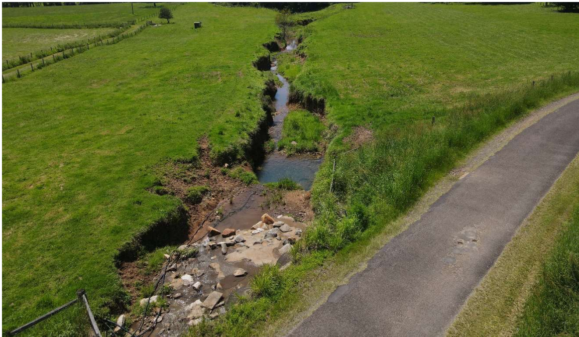
Figure 4-10. Bank erosion adjacent to Gordonville Road (JBP, 2021).
