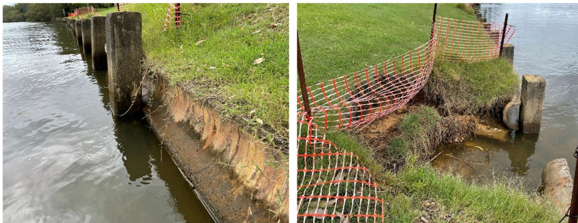
Figure 4-12. Top: Mylestom bank failures (JBP 2021).
